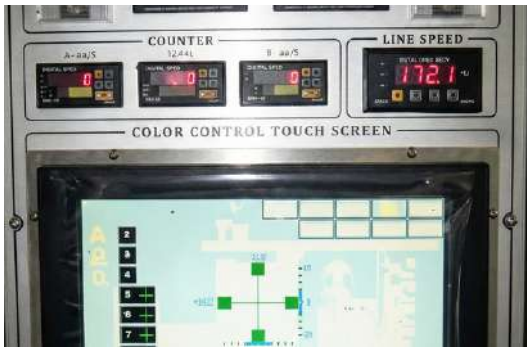
Color Control Panel
